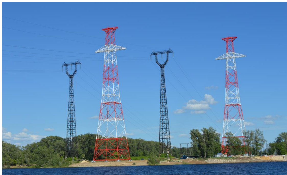
Special passage «Balakovo» 220 kV HVL across the Volga river Metal tube long-span supports, type AT-96, AT-87 ports
